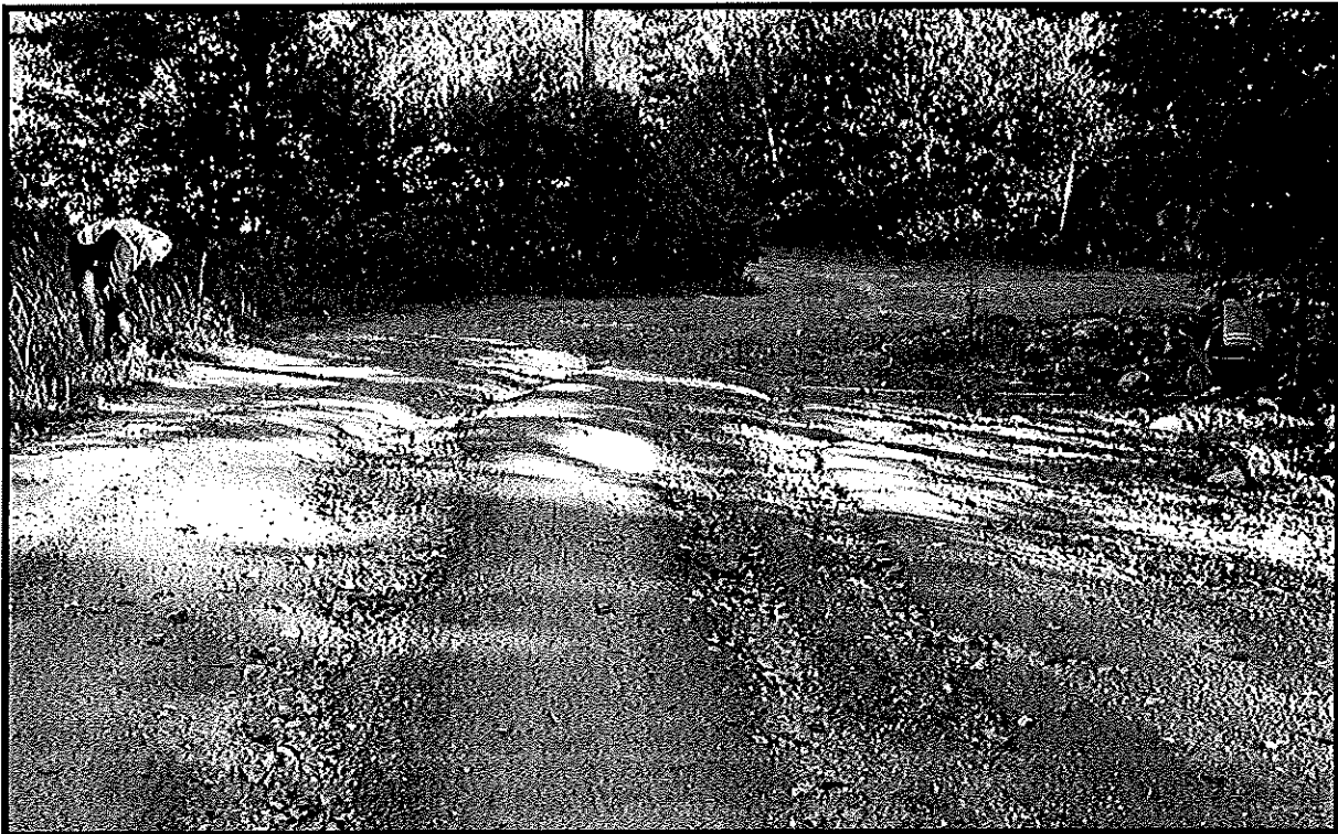
Figure 57. Erosion of roadbed. Ruts and gullies form when roads are soft in the spring and are over used. Damage can last until grading occurs.
