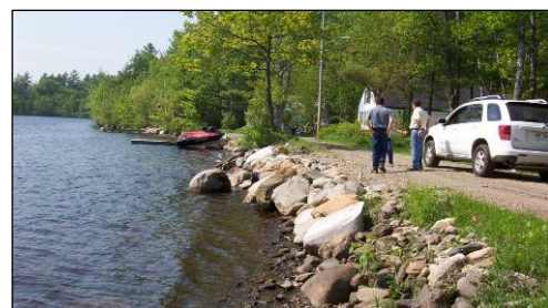
Beech Tree Drive stabilization - Hudson
