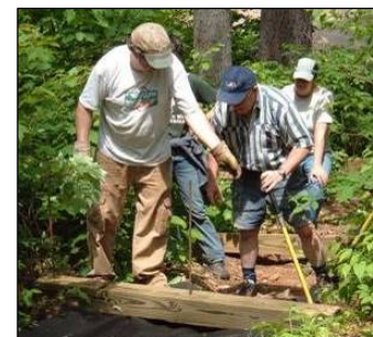
Volunteers build infiltration steps and spread mulch on an eroded path to the lake.
