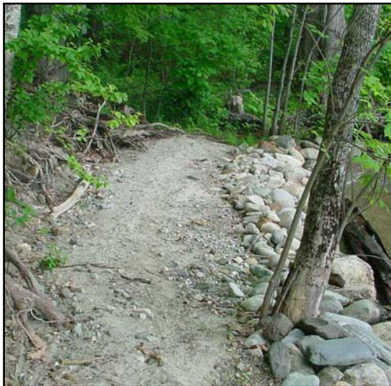
Before - Severe shoreline erosion
