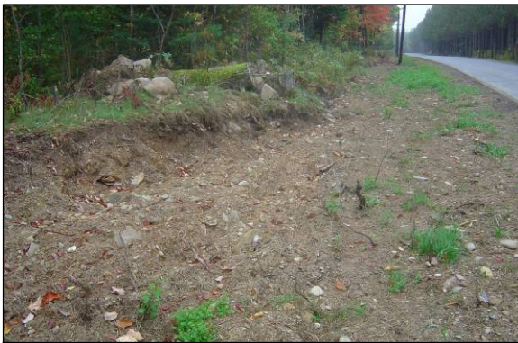
Phase I Survey, Mount Rd., Burnham - Ditch erosion/exposed soils
