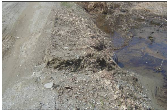
Phase II Survey, Oak Lane, Burnham - Improperly sized/installed camp road culvert
