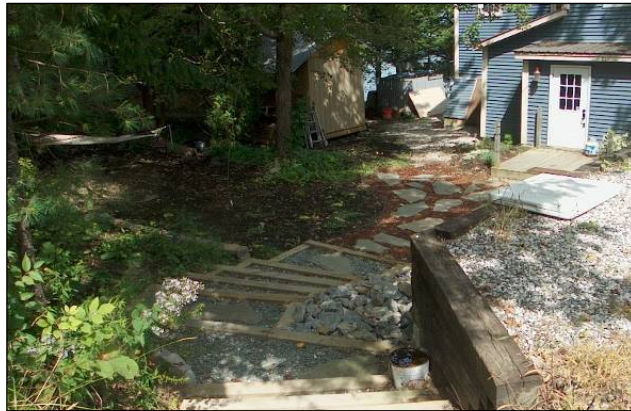
Multiple homeowner conservation practices: infiltration steps, bank stabilization and vegetation, creation and mulching of path.
