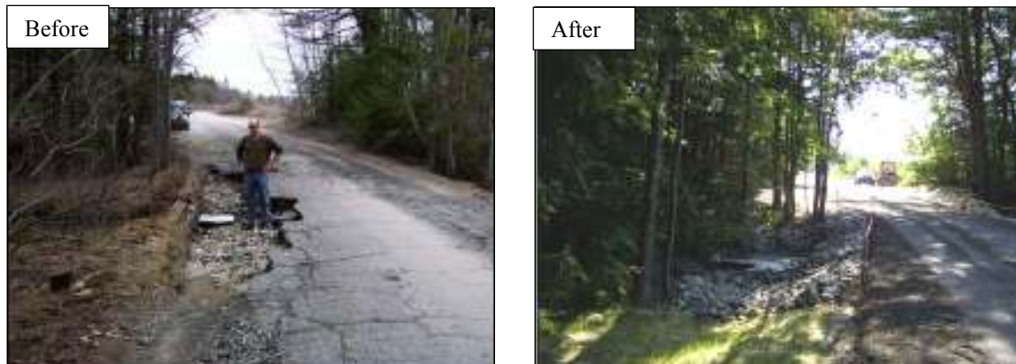
Lakeside Drive in Windham had severe road surface and shoulder erosion into a stream. Three culverts were installed to replace the two failed ones, and ditches, turnouts and new road material was installed.
