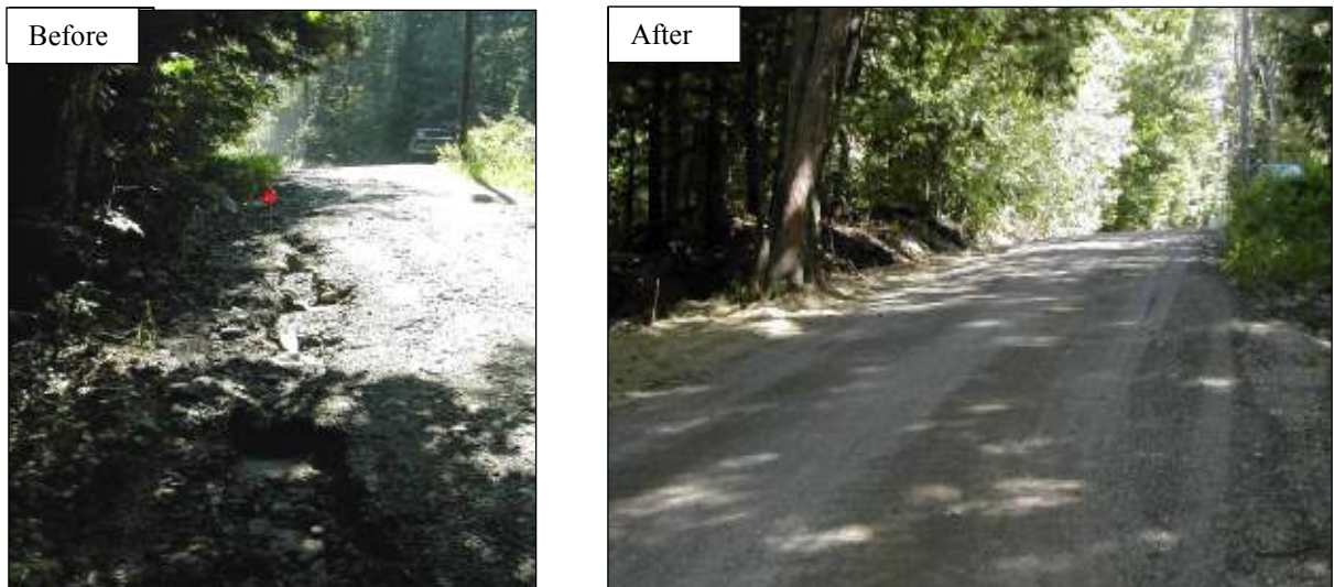
Briggs Shore Lane - Prior to improvements the site was severely eroded with deep rills and gullies carved into the road surface. Following improvements (right) the road now sheds water to a grassed ditch and plunge pools along the north side of the road.
