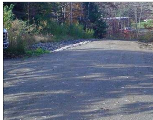
After - 900 feet of road rebuilt using BMPs to prevent sedimentation into lake.
