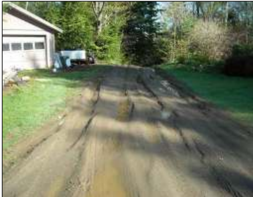
Before – Sediment from this eroding camp road washed sediment into the lake.
