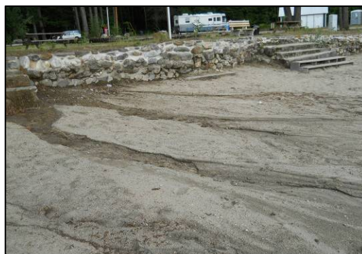
Erosion on Moy-Mo-Da-Yo Beach
