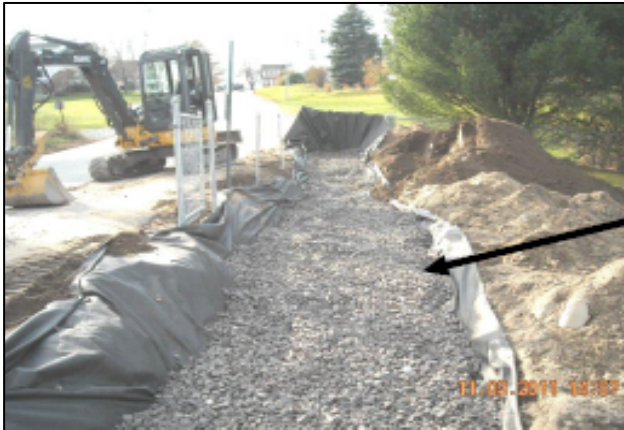
Work at Casco Town Beach included the installation of a large infiltration trench at the top of the beach (above). Straw wattles were also used to stabilize eroded shoreline areas.
