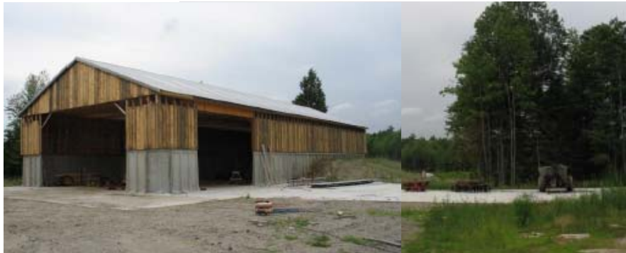
A covered, concrete manure storage facility, adjacent heavy use area and vegetated runoff treatment system were installed at a watershed dairy farm to minimize and treat phosphorus runoff.
