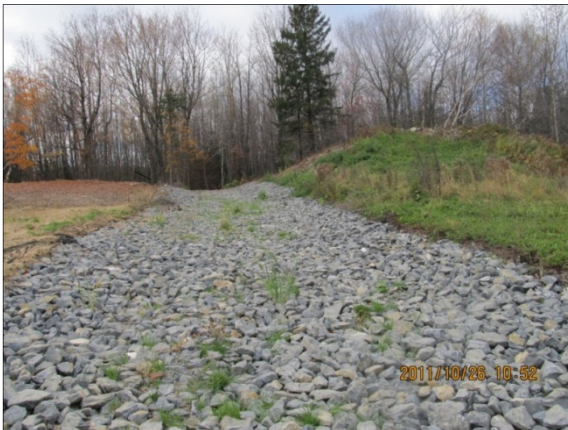
Rock-lined waterway discharging into a small pool with a level lip spreader that discharges into a riparian buffer.
