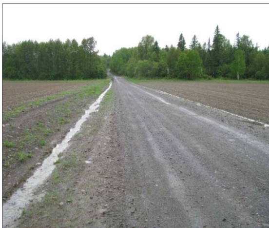
Town road lacking a stabilized ditch
