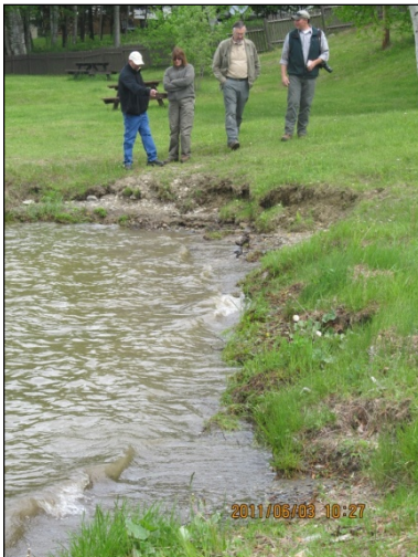
Nickerson Lake shoreline erosion before BMP installation
