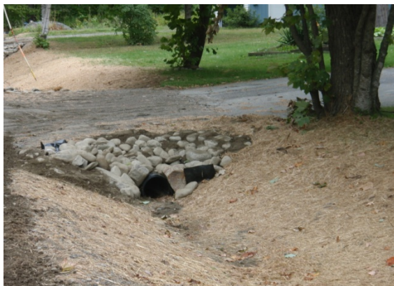
An example of a BMP installed on Woodland Ave to prevent erosion and sedimentation.
