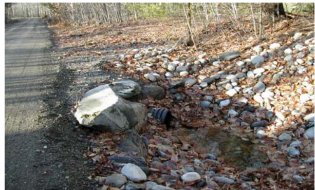
Upper Chandler Lane – After: Cross-drainage culverts installed, runoff directed into plunge pools, and surface gravel with a 6” crown was applied. Ditches were enhanced and rock-lined.
