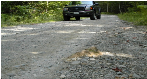
Upper Chandler Lane – Before: Ruts, shoulders severely-eroded, ditches are disconnected/ineffective.
