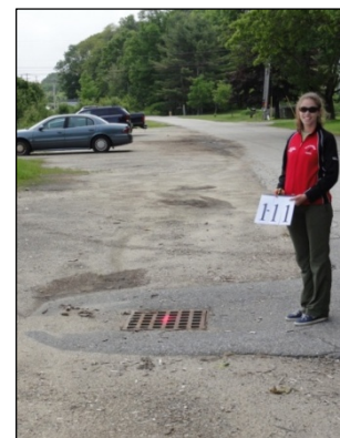
Concord Gully Brook watershed survey, eroded parking area.
