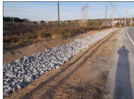
400 feet of linear ditch stabilized with filter fabric and riprap along Sylvan Road.
