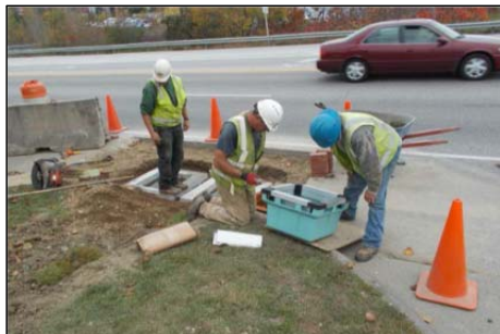
Crew installing a filter-equipped catch basin at the entrance to Swett's along Hogan Road.
