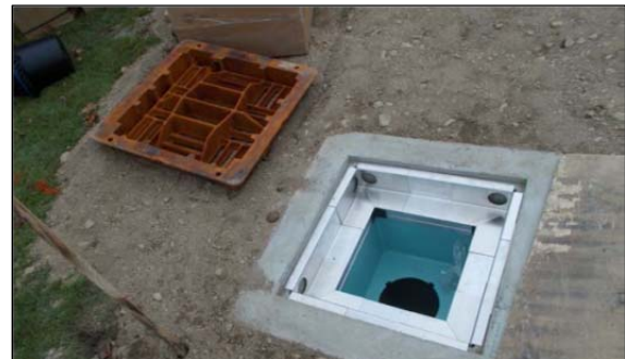
Filter-equipped catch basin installed in Swett's parking lot.
