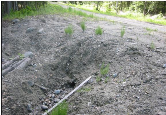
Before – Soil erosion at culvert outlet and road shoulder.
