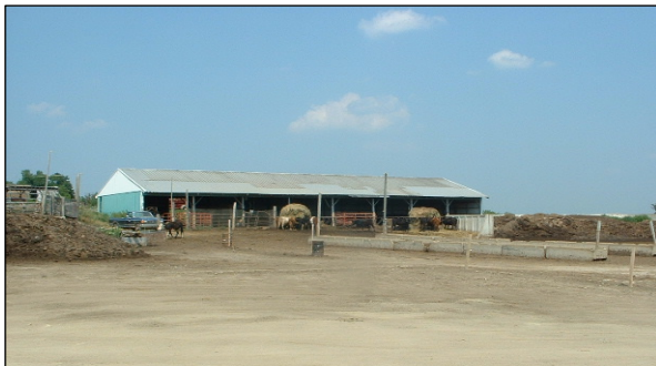
Ongoing construction on livestock waste storage and heavy use area protection pad.
