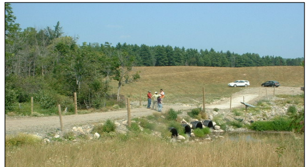
New culverts installed at stream crossing and livestock exclusion fencing along Fish Brook.
