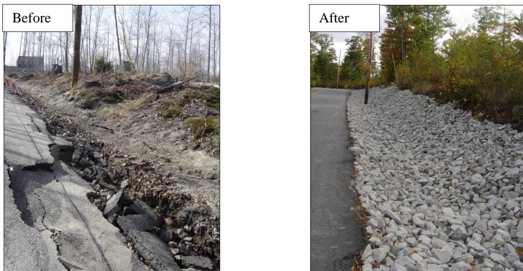
The ditch and road shoulder on Mountain View Road were severely eroded. The road shoulder was repaved, and the ditch was reshaped and stabilized with riprap.
