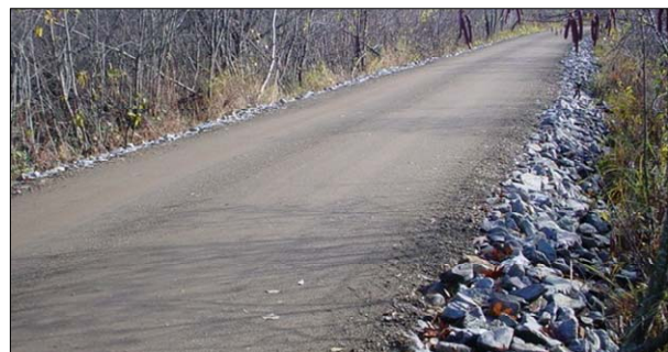
Casey Road – The causeway, which was frequently flooded and eroded, was raised and stabilized.
