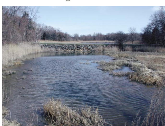
Damde Meadows salt marsh restoration, Massachusetts Two four-foot by eight-foot concrete box culverts, sized to approximate unrestricted, natural tidal flow, have replaced a failing drain-pipe that extended below two dikes.
