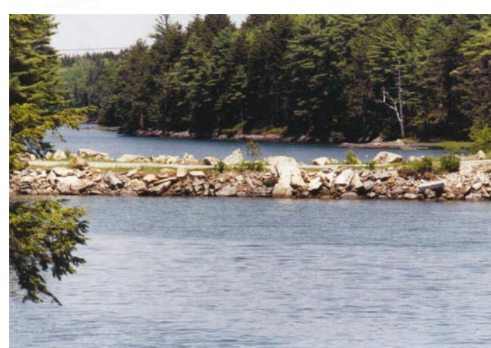
Dingley Island tidal flow restoration, Maine In 1946, the bridge connecting Dingley Island to the mainland was removed and filled. Earlier this year, a bridge span was placed in a segment of a causeway, restoring waterflow to 45 acres of clam flats. Photos: Jon Kachmar
