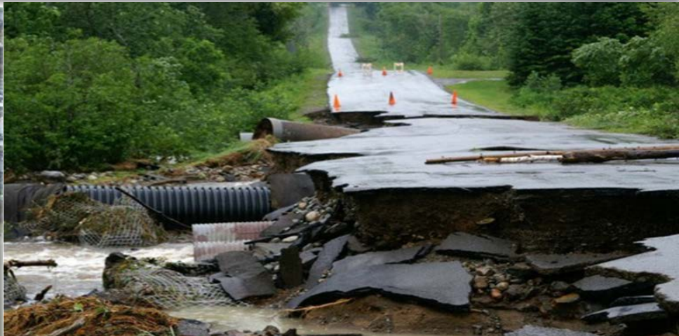
Infrastructure damage from flooding in Patten, ME, June 26, 2012. (Photo: NWS)
