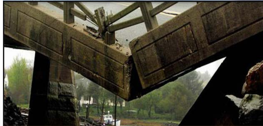
Bridge damaged above the Cape Neddick River from the May 2006 Mother's Day Floods, York, ME. (Photo: P. Wellenbach, AP)
